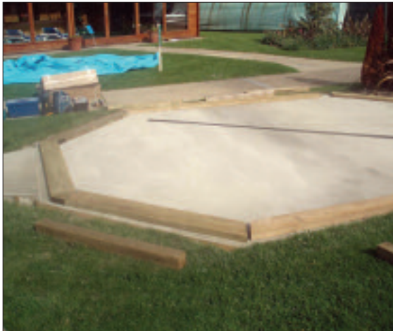
STEP 1 -Lay out the eight 200mm x 50mm base timbers on the area where the pool is to be situated.
