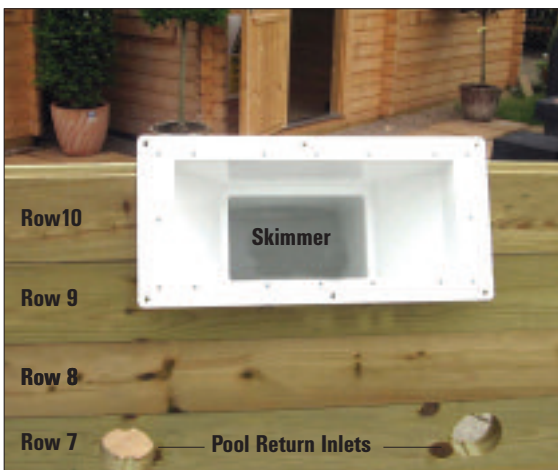
STEP 15 - Rest the skimmer on this aperture before fitting the top timber.
