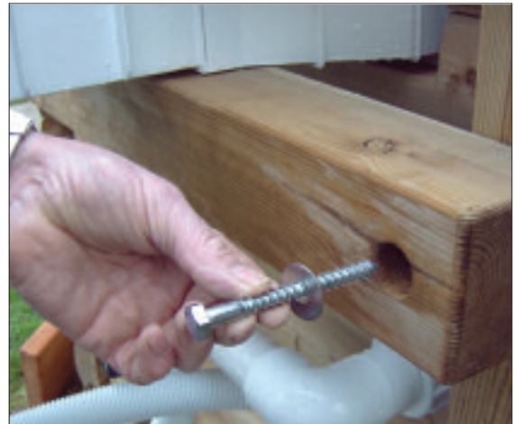
STEP 40 - Hold the skimmer support timber under the skimmer. Using the 100mm coach screws and washers, tighten with the socket wrench so that the timber supports the skimmer.
