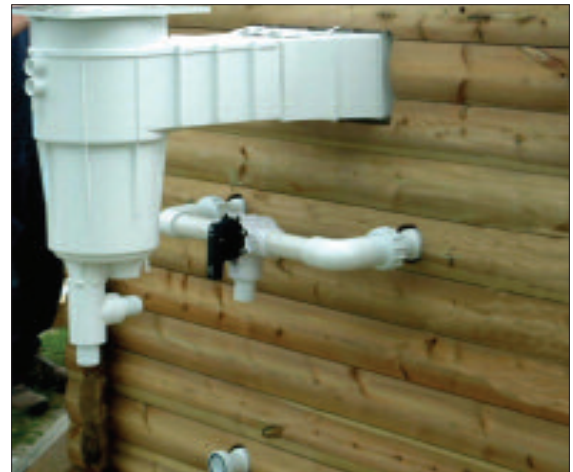
STEP 22 - The skimmer, return inlet and low suction in position. Viewed from the outside.
