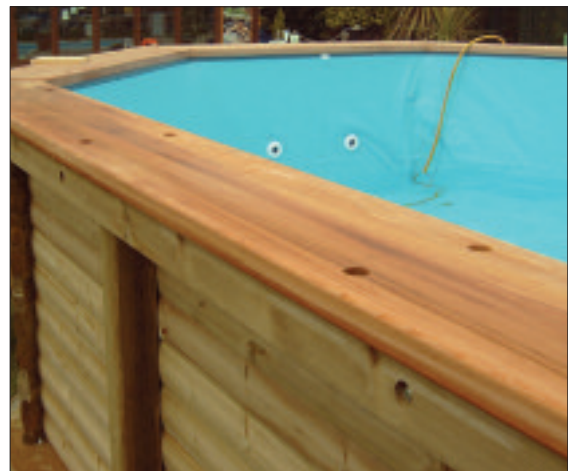
STEP 62 - While the pool is filling with water, place the timber top surround into position around the pool.
