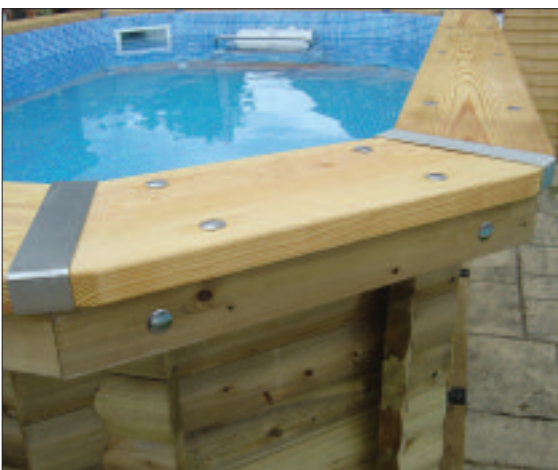
STEP 63 - Line up all 8 corners with an even overlap of the timber. Make use of the clamps to help hold the timbers into position. Using straps as per step 31, will also make this process easier.
