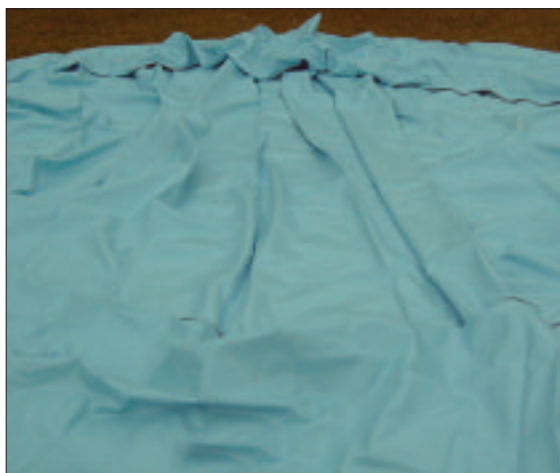
STEP 51 - Lay the liner in the pool as close to the position that the liner will be finally fitted. The liner is shaped to fit the pool, so make sure it's the correct way around. Take off your shoes when working with the liner otherwise you will mark it.
