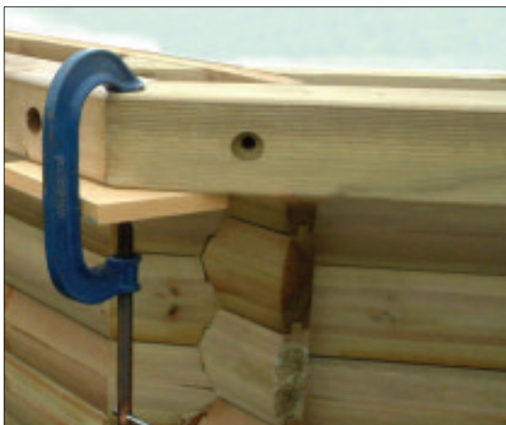
STEP 29 - Use a clamp to hold the timbers in position when drilling and fixing.
