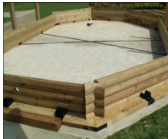
STEP 12 - Continue assembling the wall timbers, alternately aligning the corner joints. Make sure the tongues and grooves are in line before tapping down.
