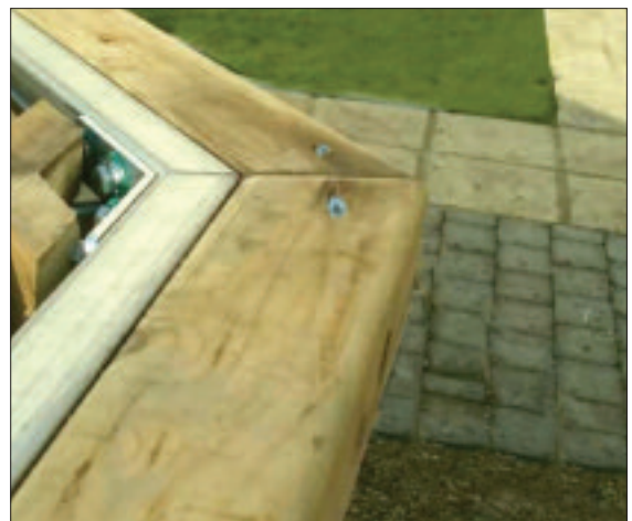
STEP 36 - The steel ring beam should lay tightly inside the timber ring beam all the way around the pool.
