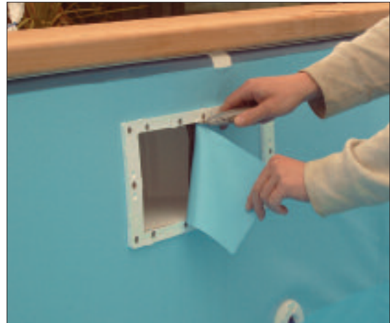
STEP 60 - Using the skimmer face plate mark the positions of the screw holes, screw on using even pressure and then cut around the inside of the plate to expose the entrance to the skimmer. Clip on cover plate to hide the screws and continue filling the pool until half way up the skimmer throat.
