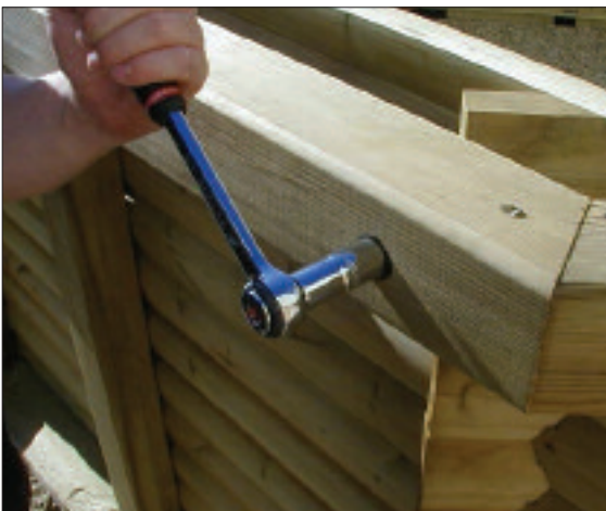
STEP 61 - Go around the pool gently tightening the nuts and checking that the pool timbers are level. Do Not over tighten.
