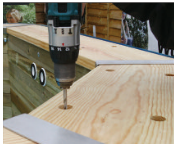
STEP 64 - When all of the top timbers are in position start by drilling a 6mm pilot hole into the timber underneath.
