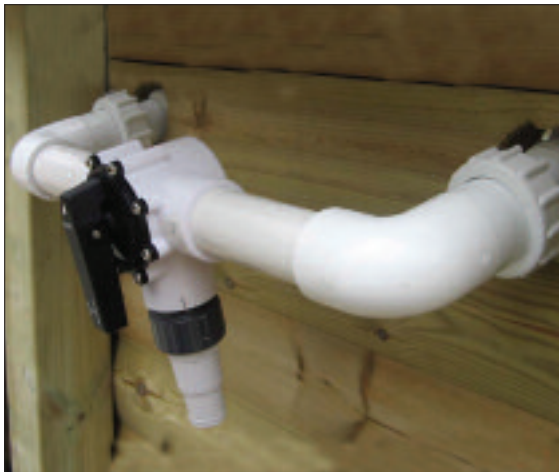
STEP 21 - Attach the return inlet pipe and valve section to the threaded unions protruding through the pool wall.
