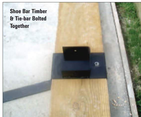
STEP 6 - Line up the shoe and tie bar - drill through the timber and tie-bar with the M10 drill. Fit the coach bolt from underneath and secure with a nut and washer.
