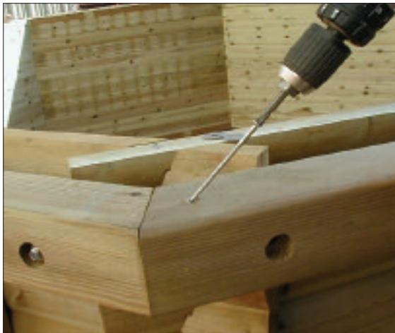
STEP 33 - Align the corners and insert the 100mm stainless steel screws as shown top and bottom making sure that the corners are aligned and level.
