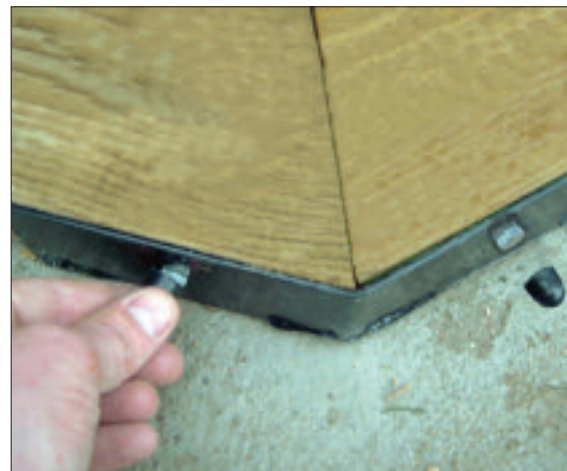
STEP 4 - Screw the 6mm coach screws into the outside of the steel corner plates. Cover the screw head with the plastic caps. Drill 4mm pilot holes if needed.
