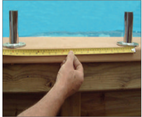
STEP 66 - Select the side where the steps are to be positioned. Stand the step flange brackets on the top surround at 500mm centres and mark the position of the holes.
