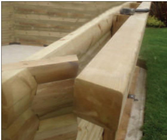
STEP 27 - Loosely attach the 96mm x 96mm timbers to the long bolts protruding through the posts. Do not tighten fully at this stage.
