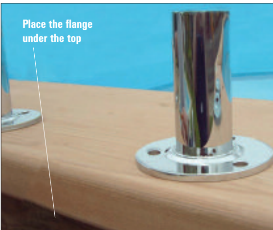
STEP 67 - Place the flange bracket so that the two holes shown are over the 96mm x 96mm timber under the top.
