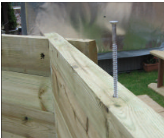
STEP 23 - Screw the half timbers to the top of the pool wall with the 100mm stainless steel screws.
