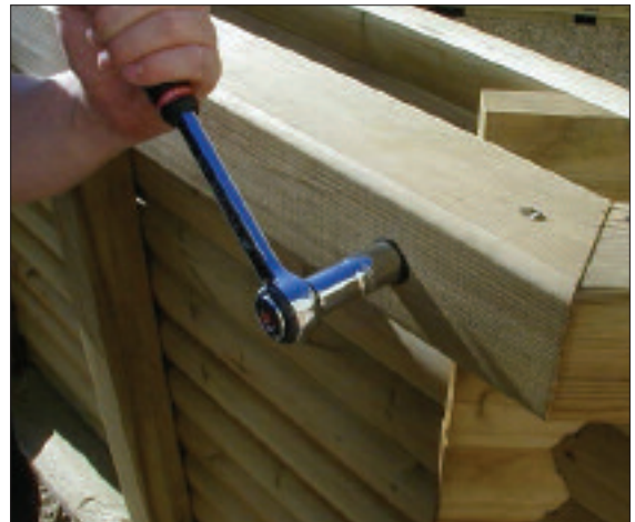
STEP 28 - Using the socket wrench firm up the nuts making sure that the washer is underneath. Do Not tighten fully at this stage.
