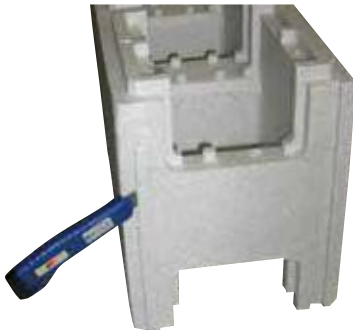
Cut the male tab of the block with a cutter, which will stop in the corner.
